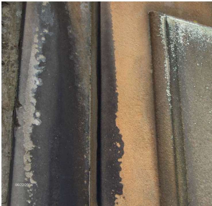
This sandstone memorial is partially covered by a hard black pollution deposit (left). The original colour of the sandstone is visible in the central area where the surface has become eroded
